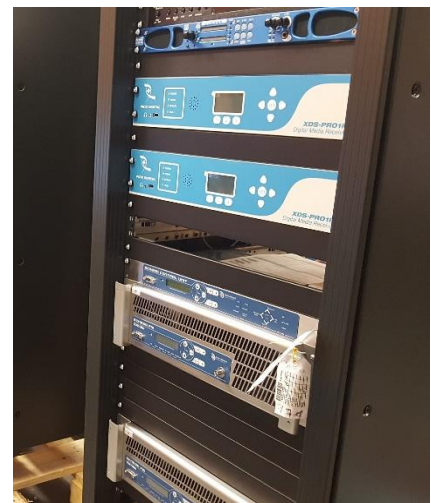
Racks of ECRESO FM 1000W in 1+1 redundancy
