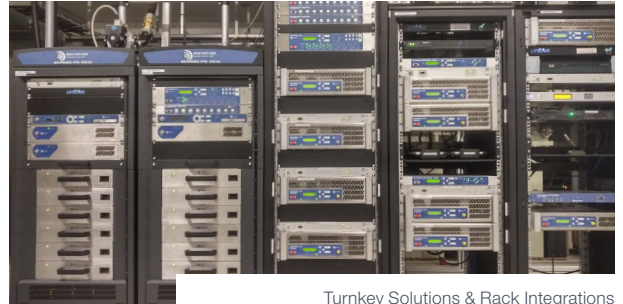
Turnkey Solutions & Rack Integrations
