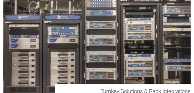
Turnkey Solutions & Rack Integrations
