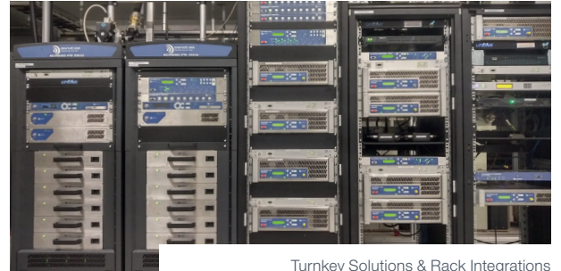
Turnkey Solutions & Rack Integrations
